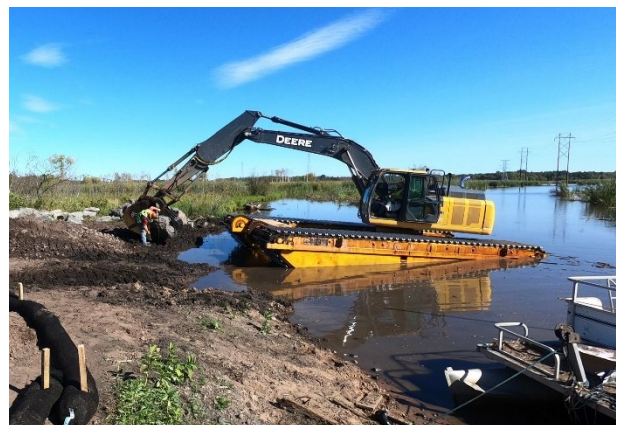
A boulder is measured during construction of a j-hook in the Kingsbury Creek inlet.
