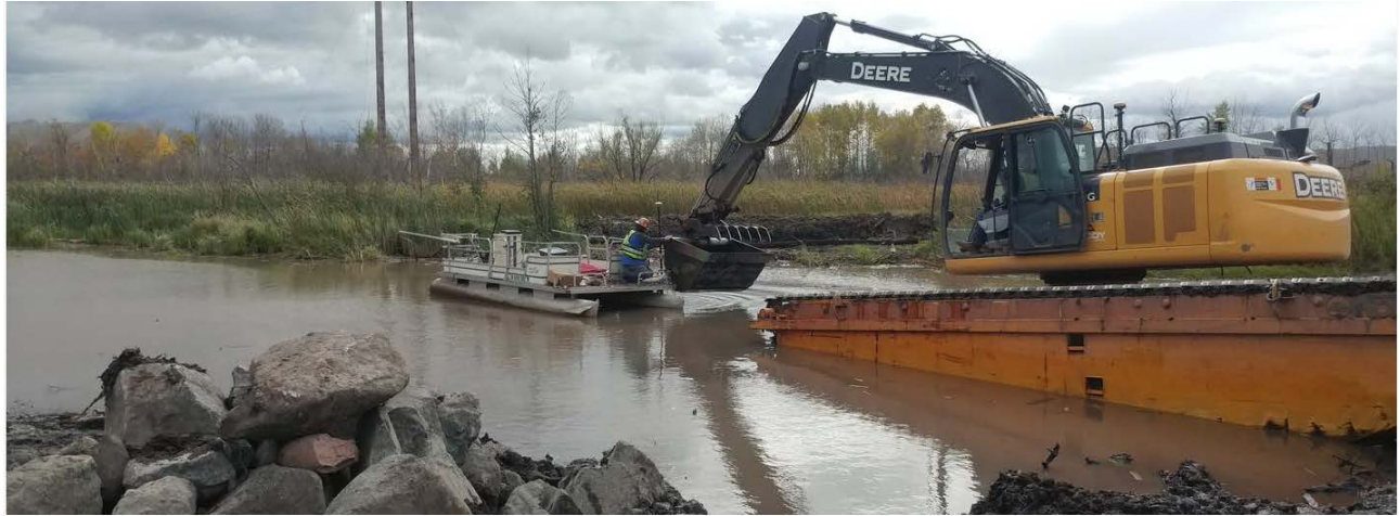
Photo Caption: A surveyor checks the location of a boulder being placed in the Keene Creek channel during J-hook construction.
