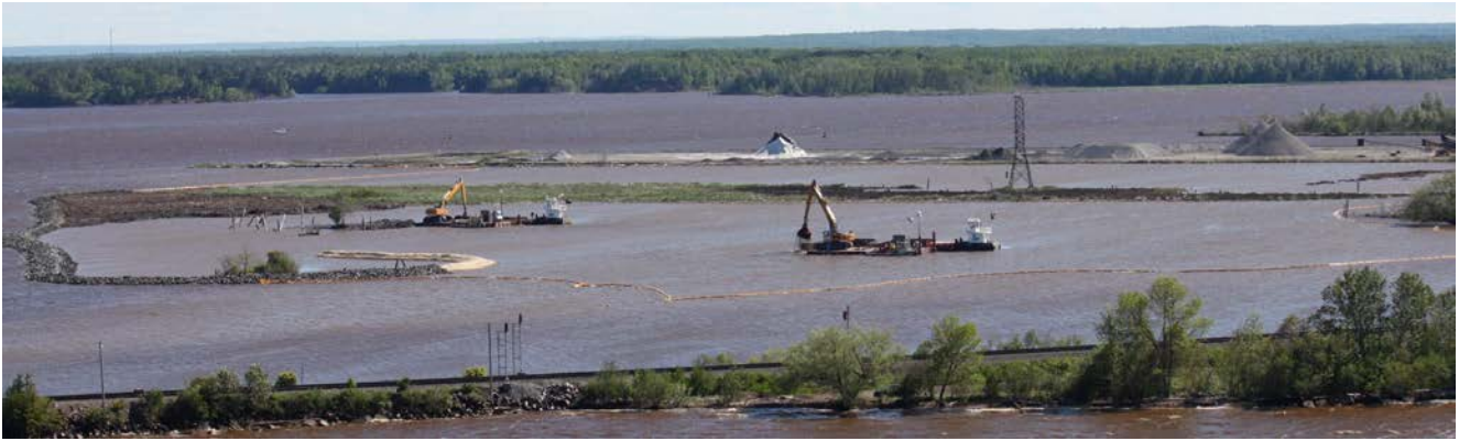
Photo: Wood waste being excavated from the waters of Grassy Point and placed to construct a new island
