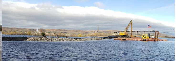
An excavator sits on a barge, placing riprap to armor the sand berm
