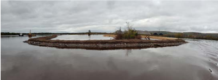
The curved sand berm at Grassy Point will contain the future island
