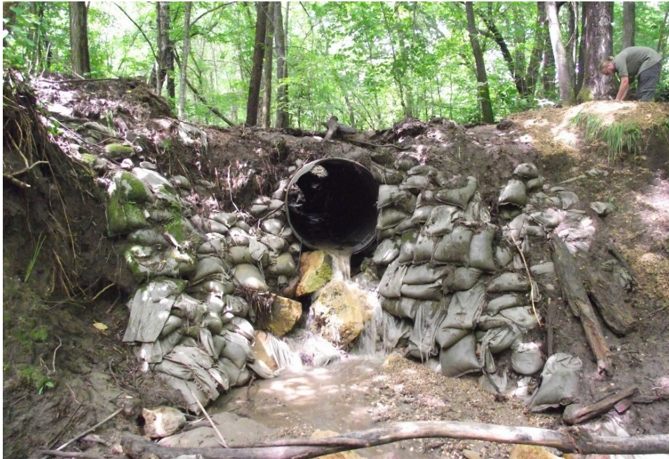
Figure B.1. Excessive jump at culvert outlet at tributary to Seven Mile Creek, Minnesota (C. Lenhart photo).
