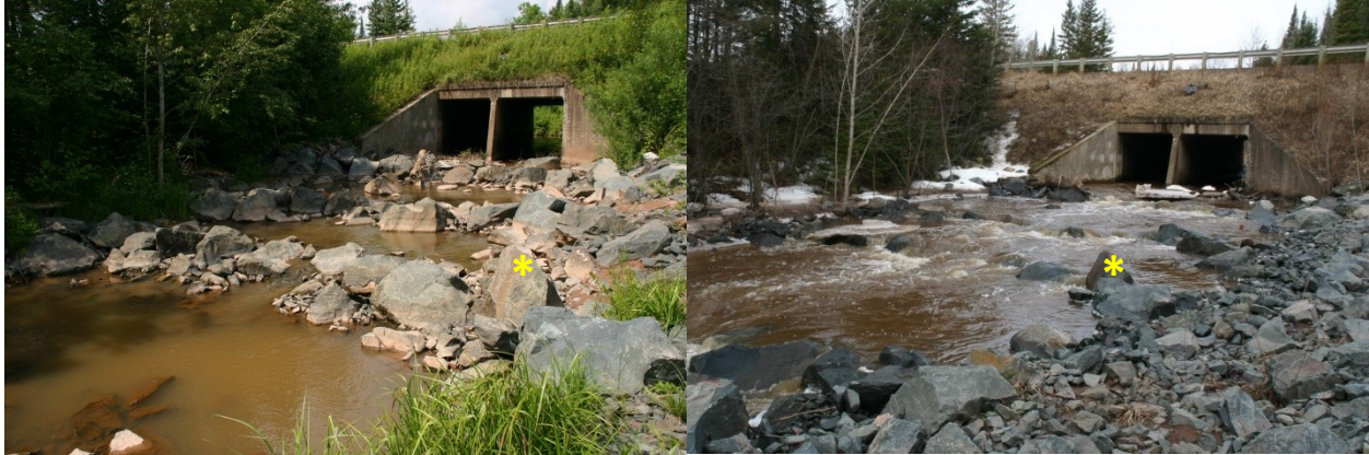
Figure 6.3.2. This series of rock weirs downstream of a formerly perched culvert (Nemadji River South Branch at TH 23 in Carleton County, see previous figure) improves passage and stream connectivity. The yellow star indicates the position of the same rock in low (left) and moderate (right) flows. Photos courtesy of P. Leete (2005).
