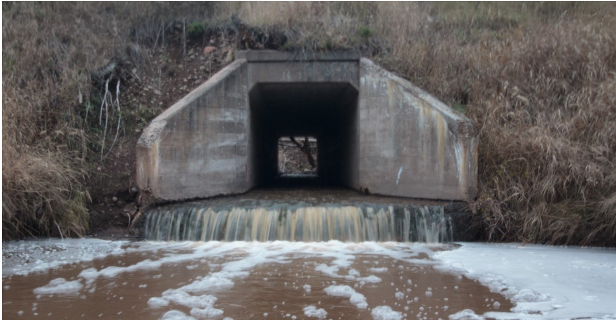
Figure 3.4.3. Perched cast in place box culvert exhibiting very shallow flow depth. Indian Camp Creek under TH61, Cook County. (P. Leete photo, 2013)
