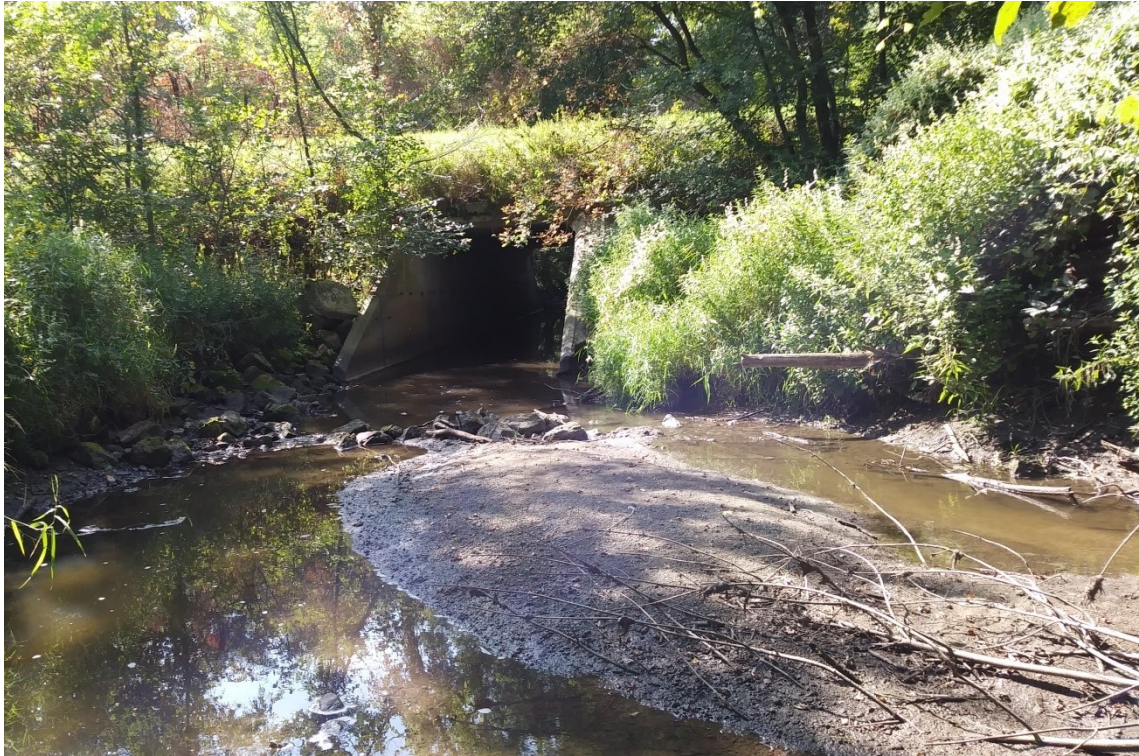
Figure 3.11.10. View of culvert inlet for Le Sueur Creek example, looking south (downstream). The east barrel on the outside of the bend conveys lower flows. The west barrel is almost hidden by vegetation growing on accumulated sediment. A mid channel bar has aggraded just upstream of a partial line of riprap.
