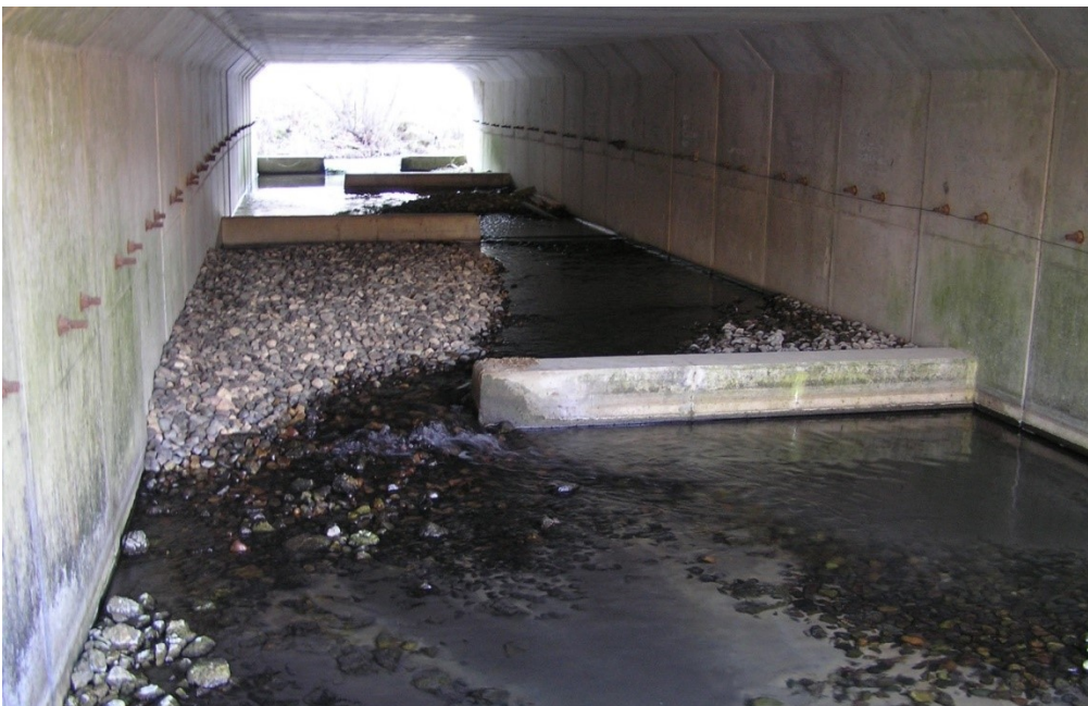
Figure 5.6.2. Alternating concrete baffles retaining gravel to cobble size material in a culvert near Red Wing, MN. Photo courtesy of B. Hansen.
