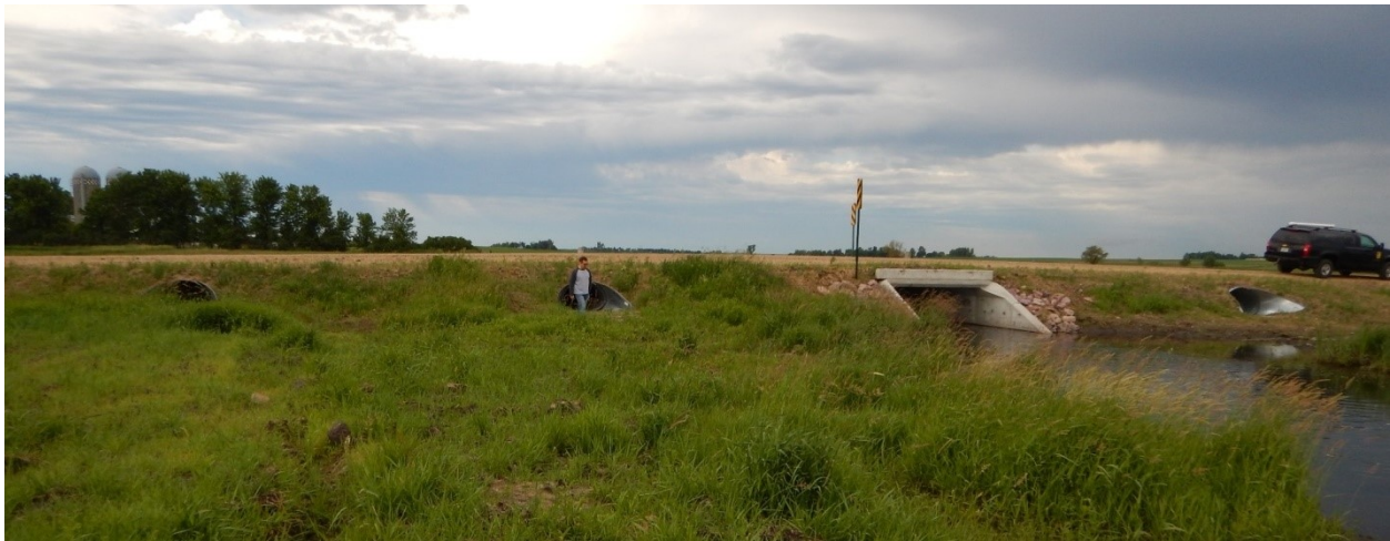
Figure 6.2.2. Three corrugated metal arch floodplain culverts flank a 12 ft x 6 ft concrete box culvert on the stream channel of a tributary to the Rock River, located in Kenneth Twp., Rock County. The on-channel culvert matches the bankfull channel width and the inverts of the floodplain culverts are set at the floodplain elevation. June 2017 photo courtesy of Kevin Zytkovicz.
