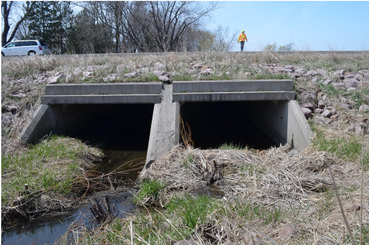
Figure 1.2.6. Aggradation at low-flow due on an unnamed stream crossing under TH 23 (bridge number 8798), Pipestone County, MN. Note the culvert width is significantly wider than the channel width. (J. Kozarek photo).
