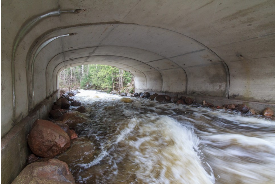
Figure 5.3.4. Swift spring flows through a culvert in Superior National Forest, northern Minnesota. Bankline rocks protect the footings from scour and simulate the bank roughness of the stream channel, allowing lower velocity regions near the bank. (P. Leete photo, 2014)
