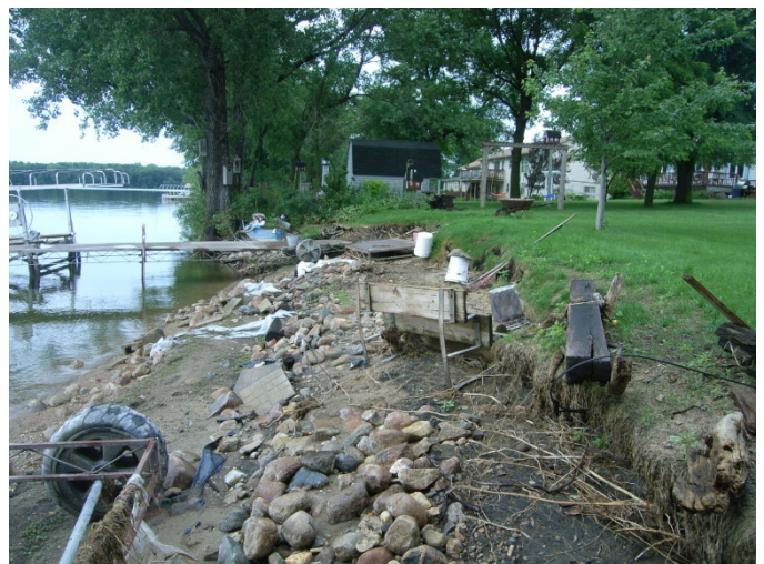
High water can overtop riprap and undermine it from behind.
