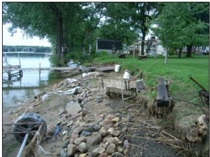
Erosion is common on waterbodies with fluctuating water levels. The establishment of adaptable deep rooted, native, woody vegetation and can prevent damage and beautify the lake. Photo credit: Murray County
