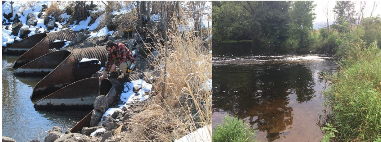
Figure 50: Photographs of the three tunnels of the culvert, in April the culverts were exposed (left) and in August they were submerged (right) showing the difference in water depth.
