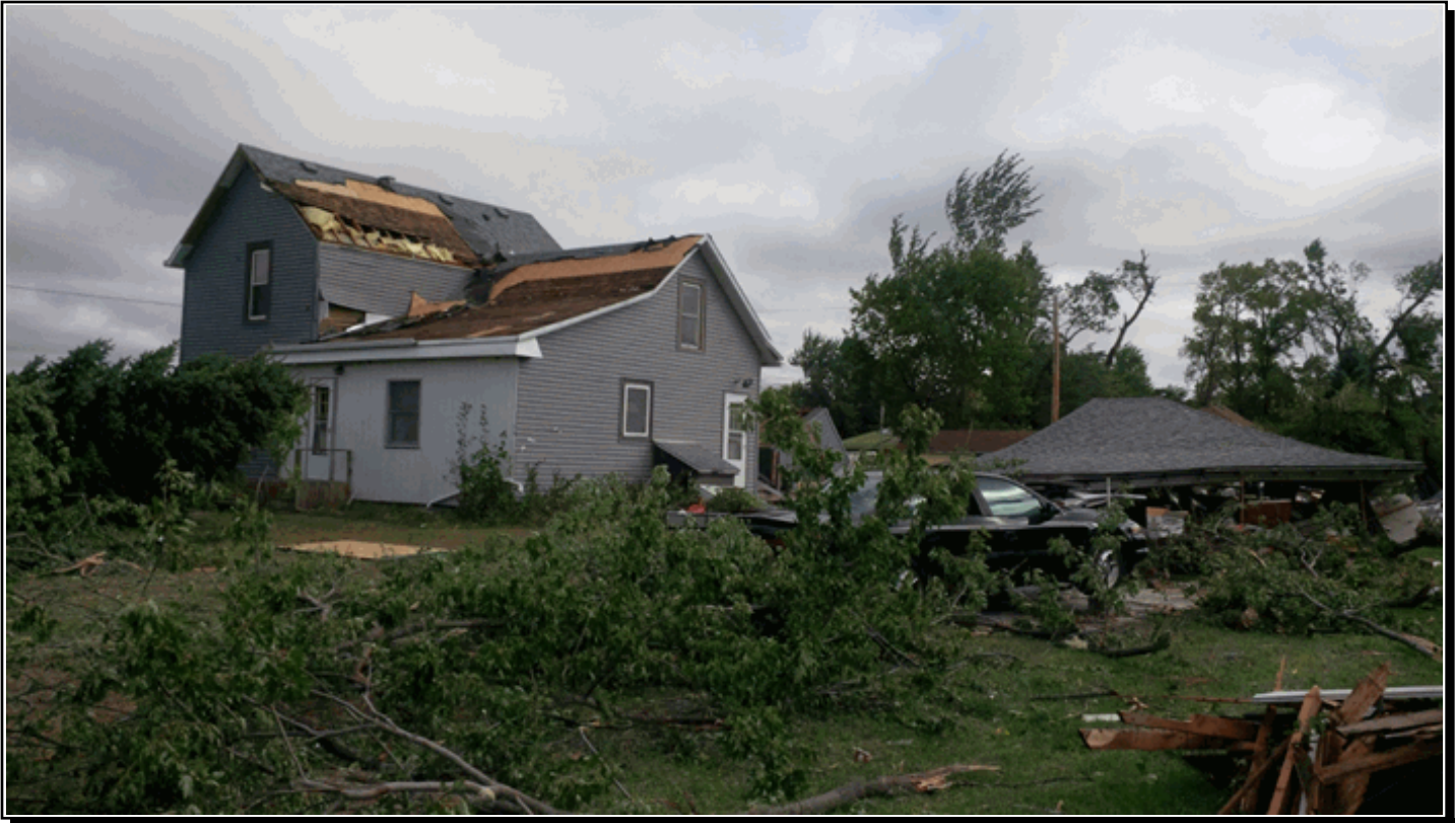
House in Granada damaged by tornado
