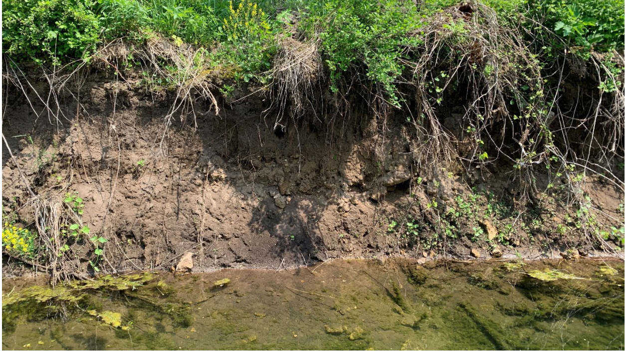
Figure 8. Eroding cutbank on west side of channel.
