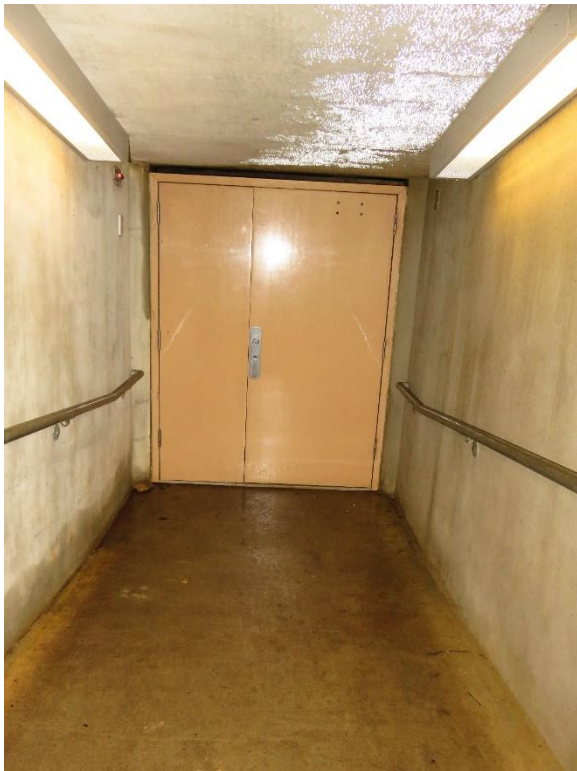
Figure 5. Second interior door at Mystery Cave Entrance 1, located in tunnel that leads to the cave.
