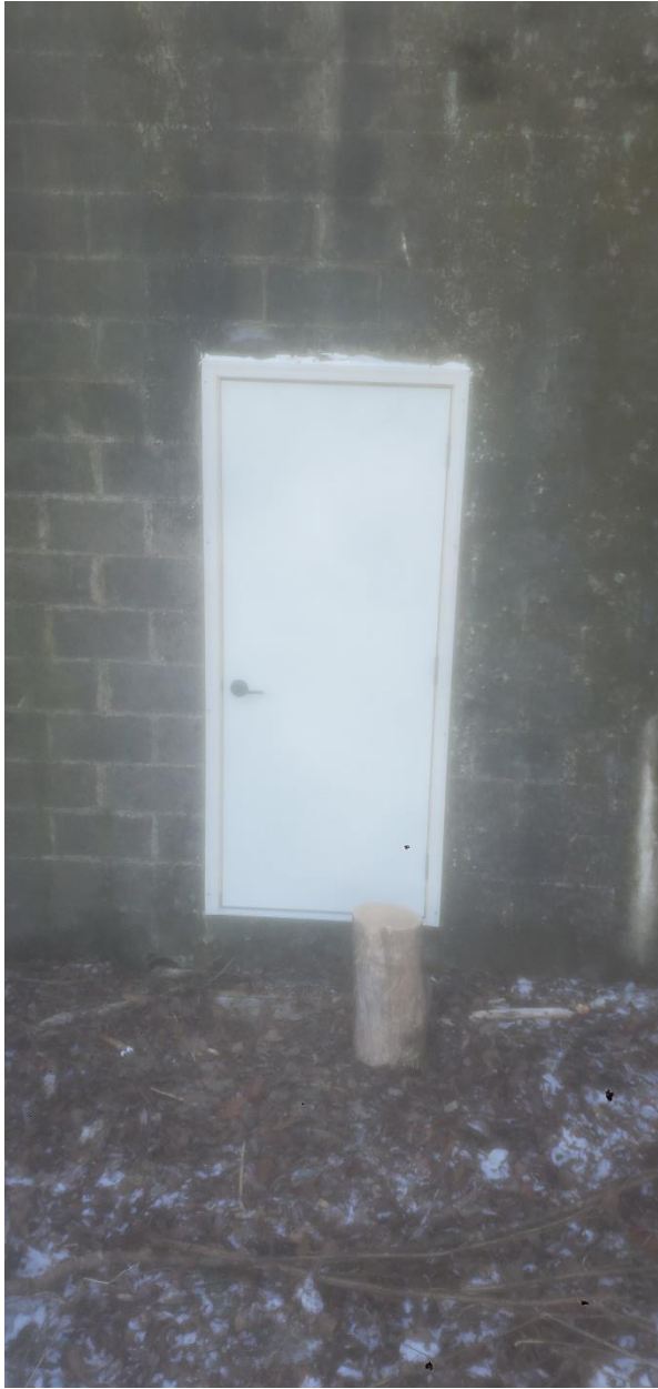
Figure 6. Exterior door for Brightsdale Tunnel. This door was replaced in fall 2024. This door replaced a previous door that began having issues staying securely closed due to weathering. Bats enter this site through a bat portal approximately 5 feet above the door (not included in image).
