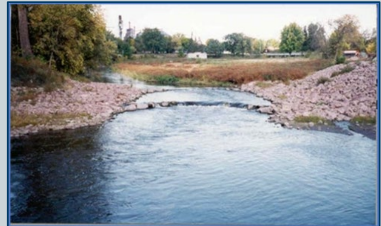
The dam was removed and replaced with a series of low-profile riffles by the MN DNR.
