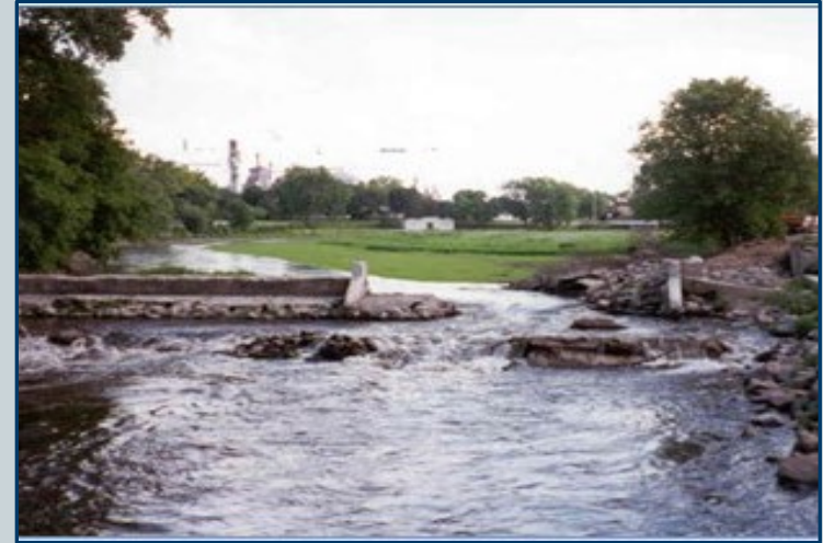
The Appleton Milldam spillway breach following flooding in April 1997.
