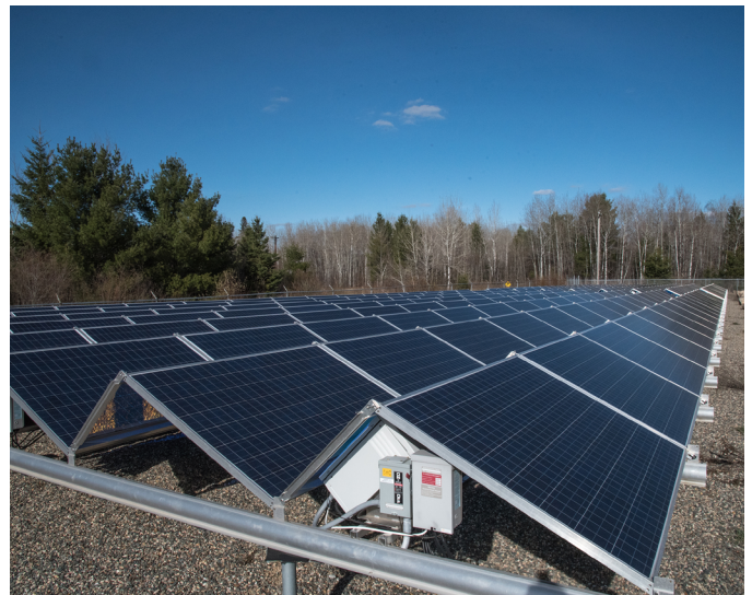
Photo: Solar panel array
