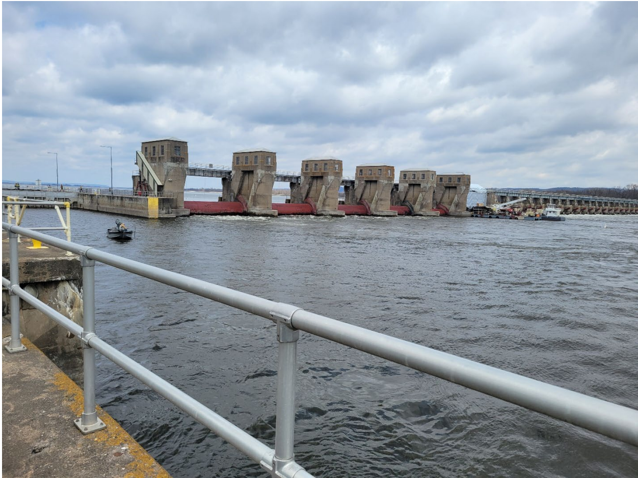
FIGURE 1.3.4-4. Roller Gates looking North
