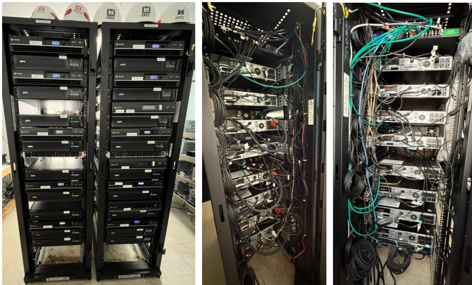
Figure 6-12. uADS Control Racks at Lock No. 19.
