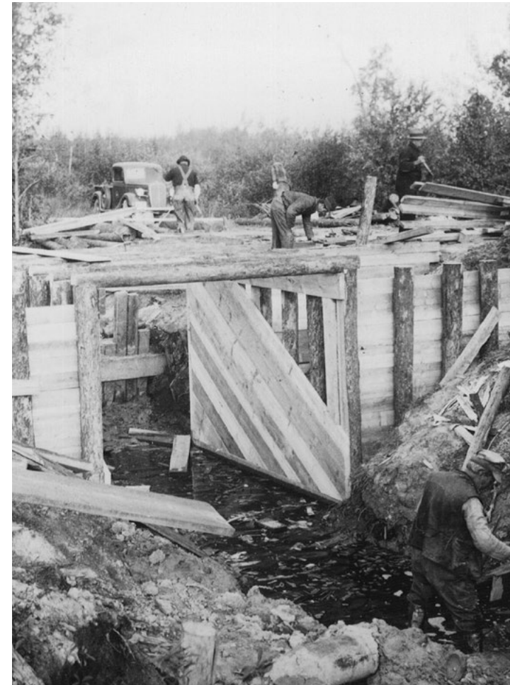
Innovative, but labor intensive, methods were used to drive piles for this dam. 1936.
