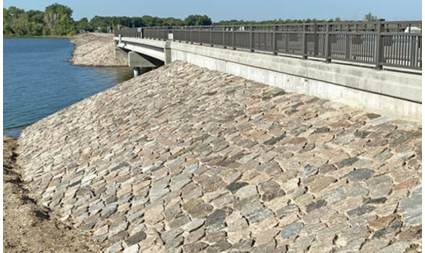
Restored stonework at the Milan Bridge. The original bridge, built in 1938, was replaced in 2020.
