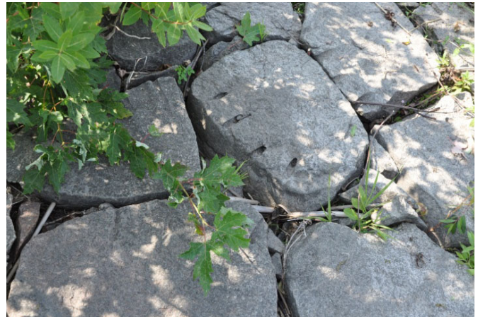
Hand-placed granite riprap at Marsh Lake Dam. Workers laid this stone riprap in many places in the Lac qui Parle Project to protect banks from erosion. Some stones have drill marks leftover from the men hand-splitting the rock.
