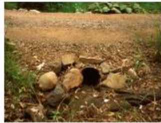
Approaches to culverts crossing drainages should be smooth and level. If the trail narrows or the shoulder is steep, place a warning sign at least 100 feet prior to the hazard.
