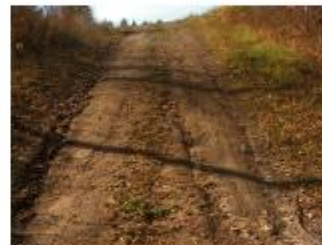
The lack of ground cover on this steeper hill is allowing erosion to take hold, making the trail unsustainable for summer use and increasingly rough for winter use.
