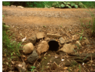
Approaches to culverts crossing drainages should be smooth and level. If the trail narrows or the shoulder is steep, place a warning sign at least 100 feet prior to the hazard.
