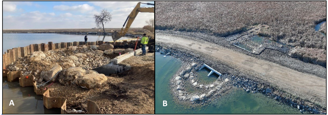
A: Construction nearing completion of the rock arch rapids. B: Final outlet structure design, showing the series of rapids acting as a 'fish ladder'.
