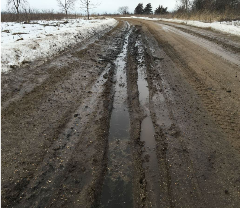
Figure 5. Example of a deteriorated state park road in need of repair.
