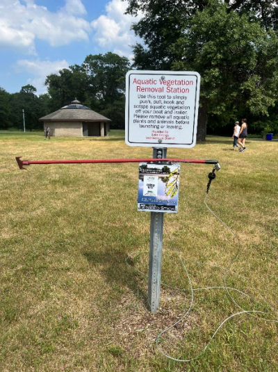
Figure 2. Cass Lake CD3 Wayside Solar Station
