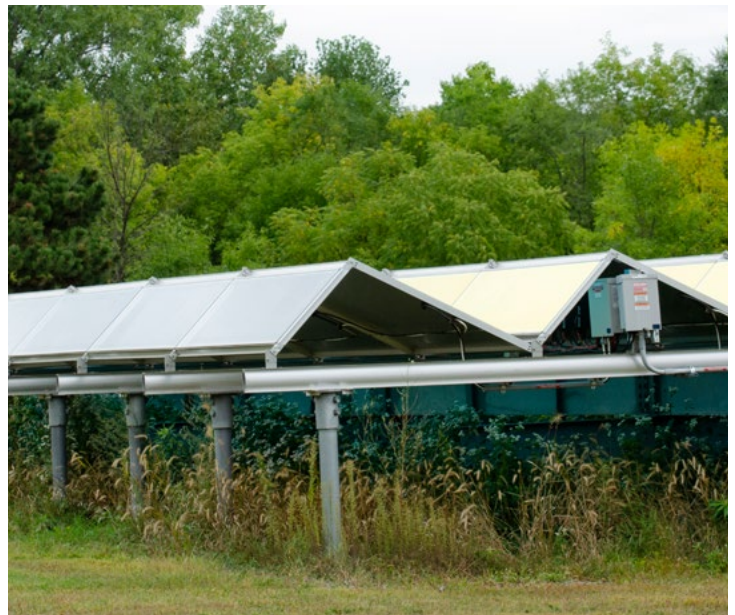
Solar panels, DNR Region 3 Headquarters
