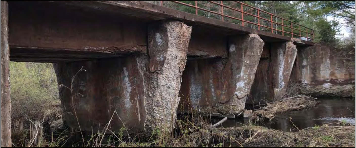
Deterioration of the Swan River Bridge.
