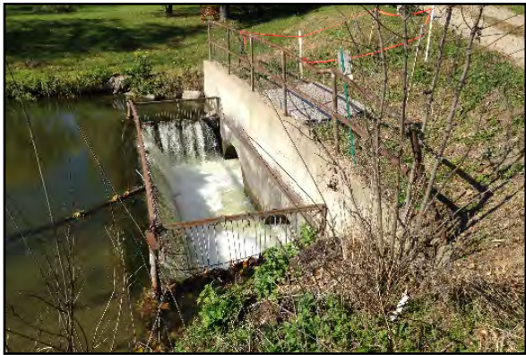
The Collinwood Lake Dam prior to rehabilitation.
