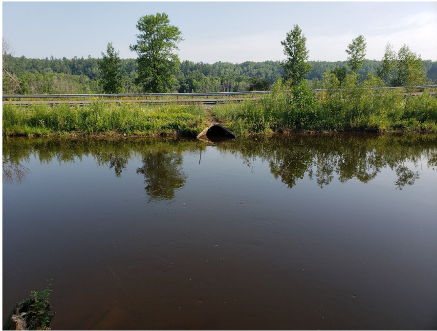
Photo 38. Looking at the existing culvert between Perch Lake and the St. Louis River via a narrow ditch. Water along with fish and other aquatic organisms, sediments, and nutrients are required to pass through this narrow pipe as the only connection. The newly installed culvert will be approximately four times wider than this culvert. Photo taken by M. Pranckus (EOR) on August 18, 2023.
