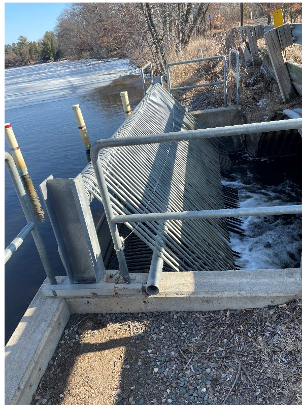
Photo 45. Martin Lake outlet barrier, photo taken during site visit 3/1/24.
