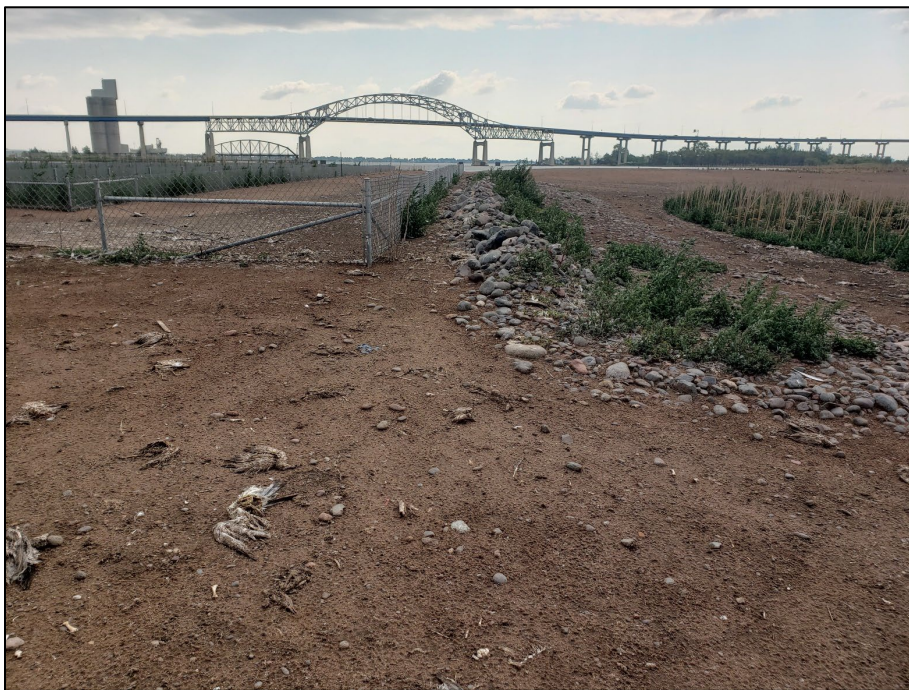
Photo 19. Looking the nesting fence structure along with a rip rap berm intended to reduce wind erosion on Interstate Island. Photo provided by M. Pranckus (EOR) 8/17/2023.
