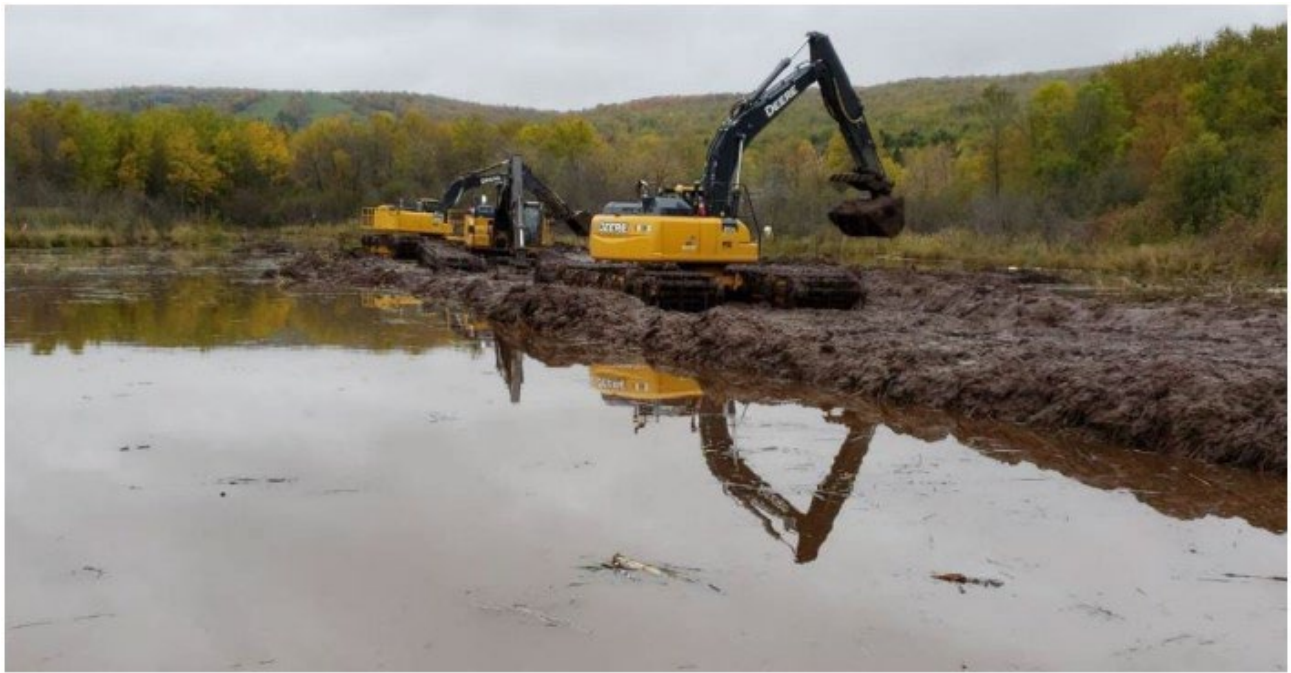
Photo 26. Example of excavation activities to removal cattail vegetation for off-site disposal at Kingsbury Bay. Photo provided by MNDNR Lake Superior and St. Louis River Program.
