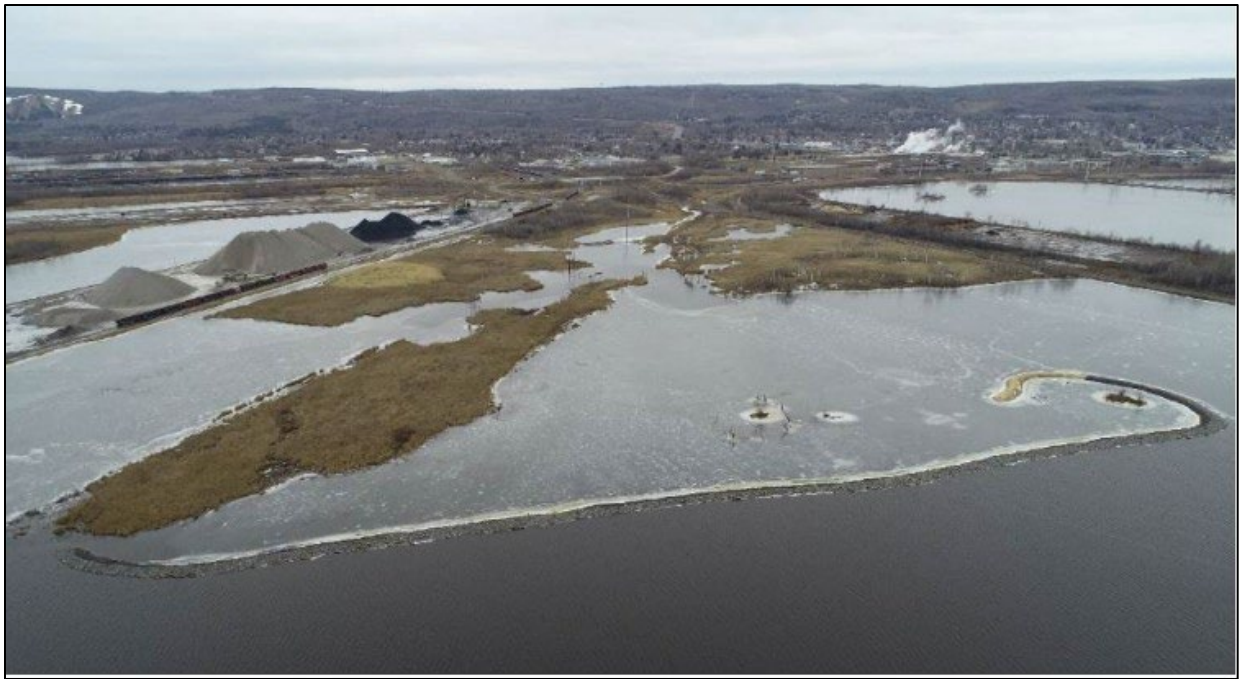
Photo 3. Aerial view of island construction at Grassy Point. A stone berm was established on the shoreline adjacent to the main St. Louis River channel to reduce erosion and set the perimeter. Photo provided by MNDNR Lake Superior and St. Louis River Program.
