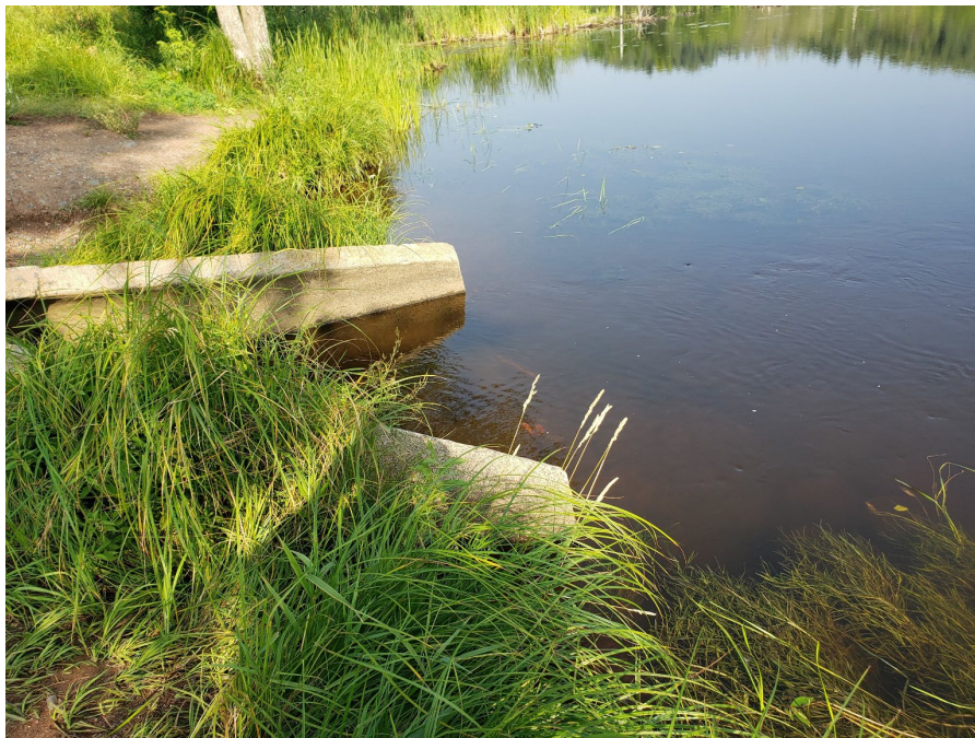
Photo 37. Example of the existing culvert outlet connecting Perch Lake with the St. Louis River. This culvert will remain in place following the installation of the new culvert at a second location under State Highway 23. Photo taken by M. Pranckus (EOR) on August 18, 2023.
