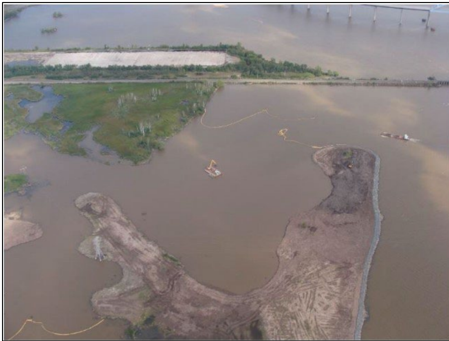
Photo 5. Aerial view of operations to place material excavated from Kingsbury Bay as a biomedium within the open water portions of the Grassy Point wetland complex. Photo provided by 1854 Treaty Authority via MNDNR Lake Superior and St. Louis River Program.
