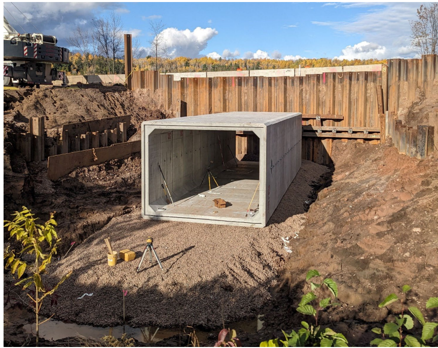
Photo 40. Installation of the new culvert connecting Perch Lake with the St. Louis River. The photo was taken after the initial site assessment visit. Photo provided by Jeramy Pinkerton, MNDNR.
