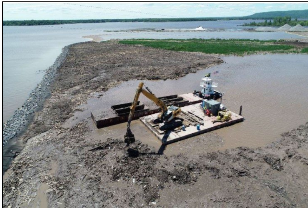
Photo 4. Example of wood waste excavated from the portions of Grassy Point that were deepened to restore the open water wetlands to a bathymetry similar to reference conditions being installed to build one of the two islands being created for the project. Photo provided by MNDNR Lake Superior and St. Louis River Program.
