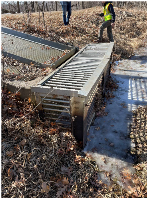
Photo 43 Barrier with retrofit at inlet of Bone Lake, photo taken during site visit 3/1/24.
