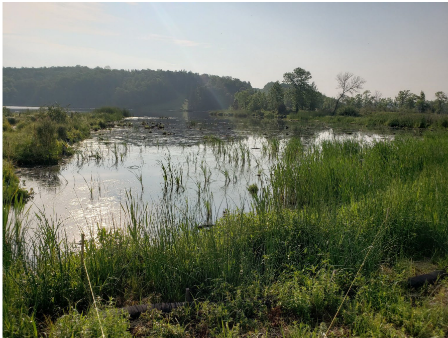
Photo 41. Example of the equipment access pad post-construction. Timber mats were placed on wetland vegetation to minimize impact during construction. Photo taken by M. Pranckus (EOR) on August 18, 2023.
