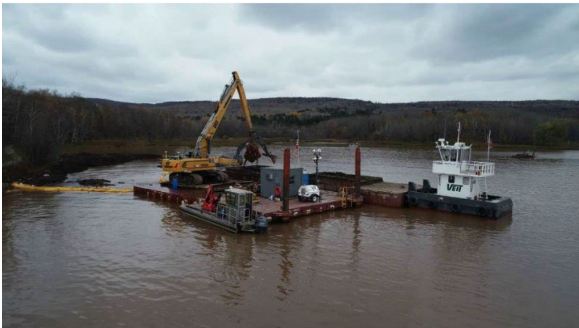
Photo 27. Example of excavation activities to removal accumulated sediment following cattail vegetation removal at Kingsbury Bay. Material was loaded in a barge and deposited at the Grassy Point restoration site on the St. Louis River. Photo provided by MNDNR Lake Superior and St. Louis River Program.
