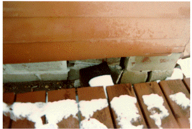
The foundation of this cabin on Big Cormorant Lake suffered damage when ice jacking jammed an unattached deck into the foundation block.
