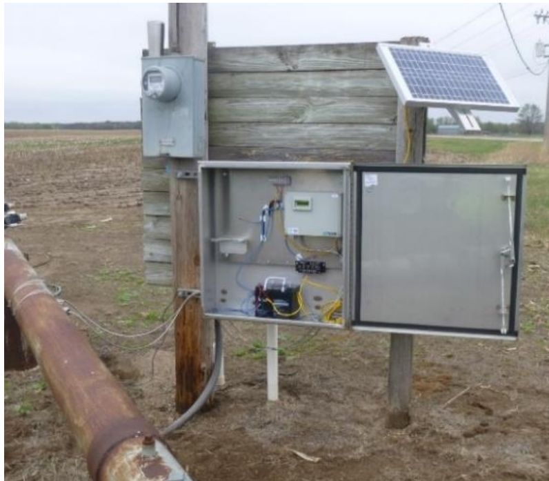
Figure 3 – Flow meter gage house set up
