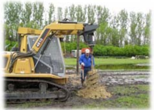
Figure 2. Holes are drilled using an ASV or skidsteer with a 4’x12” auger and 24” extension. Corner, gate and brace posts are set 6’ deep and line posts are set 4’ deep.
