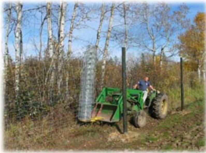
Figure 8. To unroll wire, the wire spooler is attached to a loader bucket using load binders. The wire is tacked up temporarily as it is unrolled.
