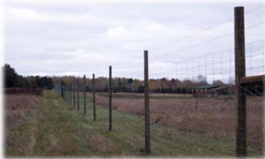
Figure 10. A typical fence line with line posts spaced at 20 ft., and two horizontal strands of smooth wire strung above the woven wire.
