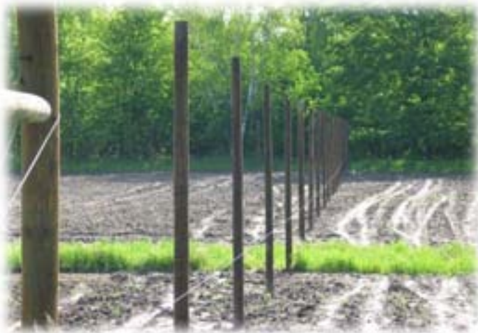
Figure 3. High Tensile wire, strung 3' above ground and stretched from corner to corner, aids in post layout and alignment.
