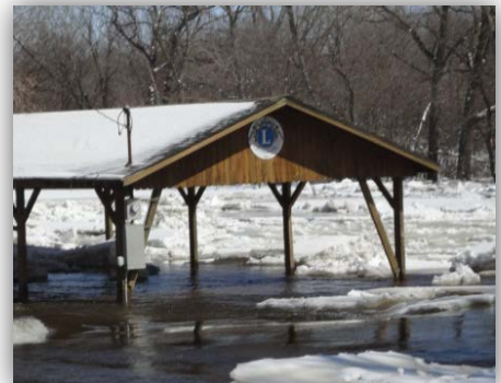
Figure 2 (below): same structure later allowed floodwaters to pass through.
