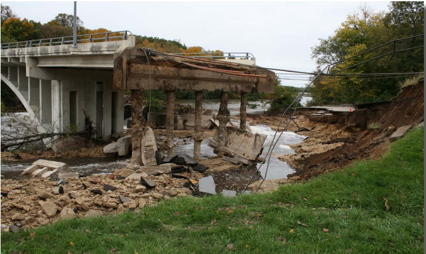
Aftermath of the Shady Lake Dam break near Oronoco in Olmsted County
