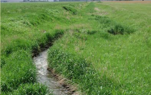
This ditched stream has been allowed to re-establish a meandering channel between ditch banks. Lawndale Creek, Wilkin County.
