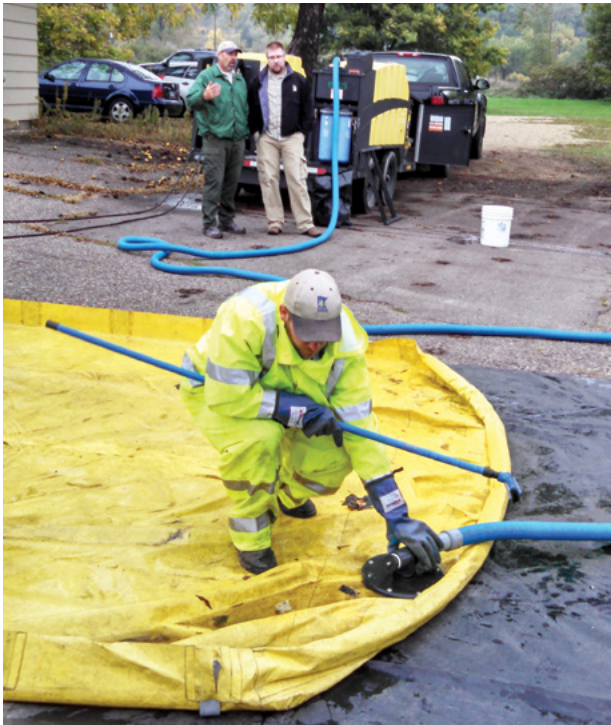
Inspector reclaims water from mat using the vacuum head attached to vacuum hose.
