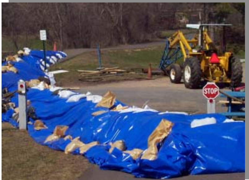
Levee closure across a road opening in Afton
