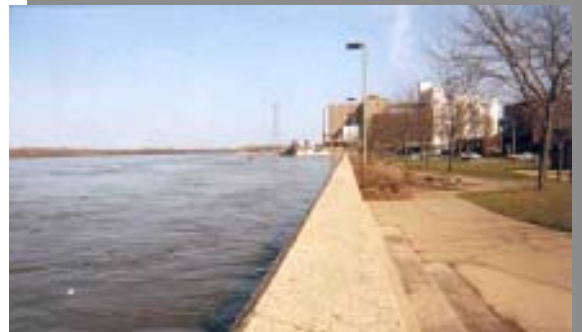
Winona flood control structure built in the 1950s with help from the Corps (shown in 2001)
