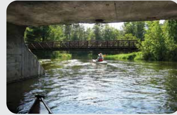
Be alert for box culverts and low culverts at the beginning of this water trail.
