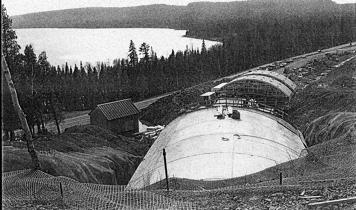
Construction of Lafayette Bluff Tunnel on TH 61. Photo by Lee Radzak , Minnesota Historical Society.
