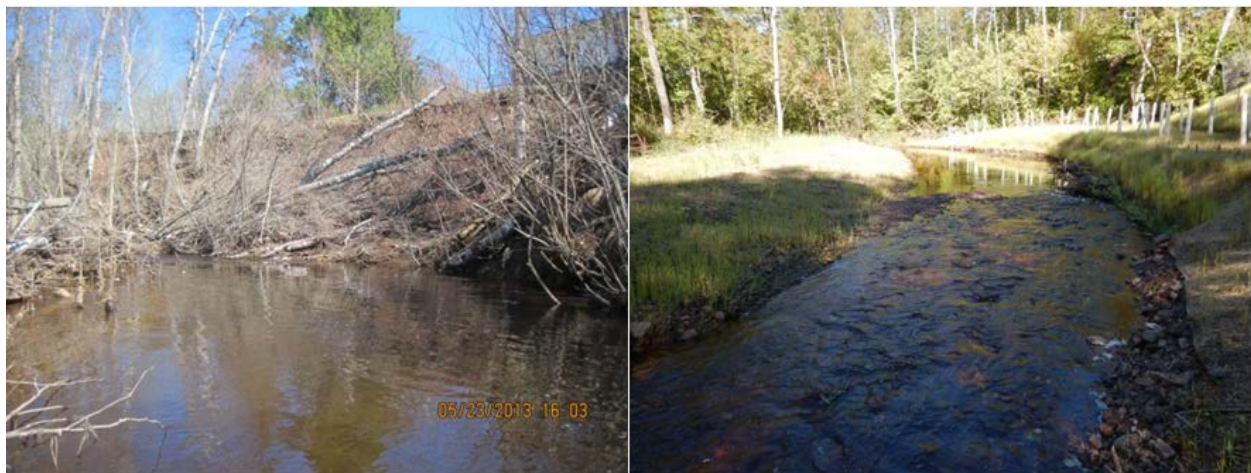
Photos: The 2015 South St. Louis SWCD bank stabilization project on East Amity Creek, upstream of Jean Duluth Road, before (left) and after (right) completion. Photo credit: South St. Louis SWCD.
