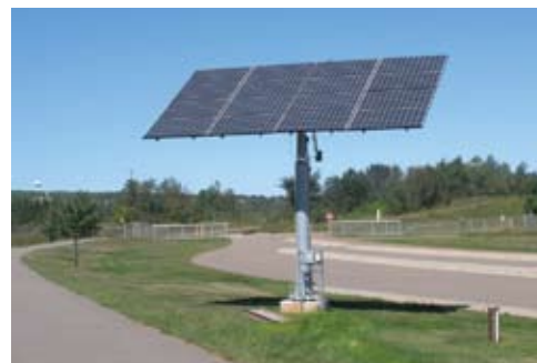
This photovoltaic array at the Iron Range OHV Recreation Area tracks the path of the sun, producing over 5,700 kWh per year.
